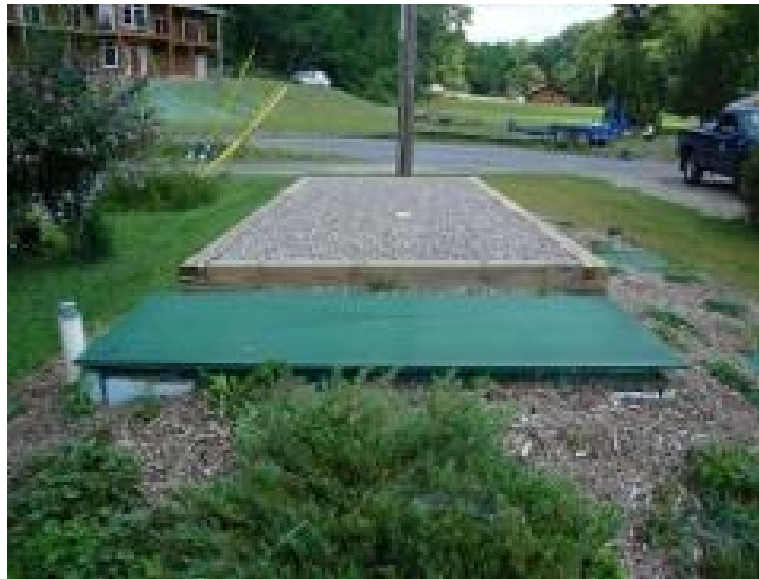
Figure 3. Decentralized ETUs: Orenco AdvanTex with Sand Filter
