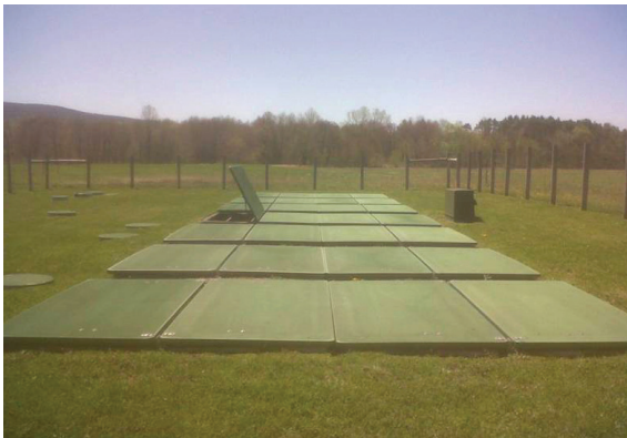
Small Community Cluster System (SCCS) treatment area for Hillsdale, NY showing seven textile filter based media ETU's.
