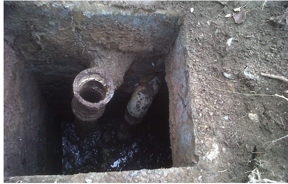
View into the top of a failing septic tank in Westchester County with concrete material corroded away and the tank is no longer water-tight.
