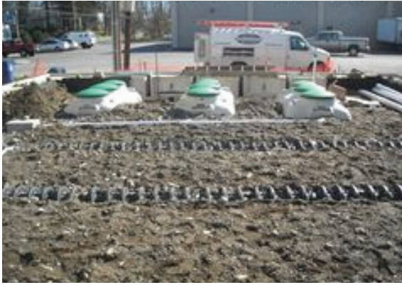
Installation of a commercial ETU system using fixed plastic media for treatment on a small lot serving a large three floor building with a restaurant & pub on the ground floor and residential apartments on the upper floors.
